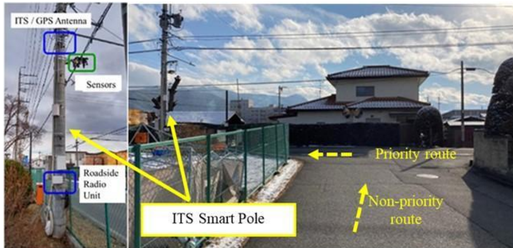
FIGURE 7.13 The target non-line-of-sight intersection and the installed ITS Smart Pole
